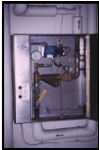
Fig. 2-10. Valve junction panel.
